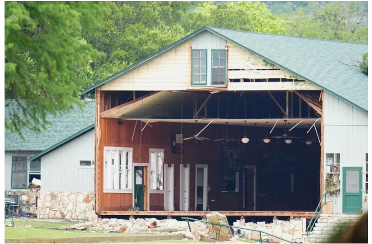
A full wall is missing from a Camp Mystic building after the Texas floods. The building is located near the Guadalupe River, where water rose over 20 feet during the flooding and affected many other buildings on camp property. Photo courtesy of Julio Cortez and AP Photo.
